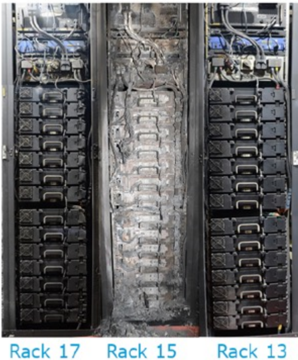
Figure 13: Destruction of Rack at McMicken.
