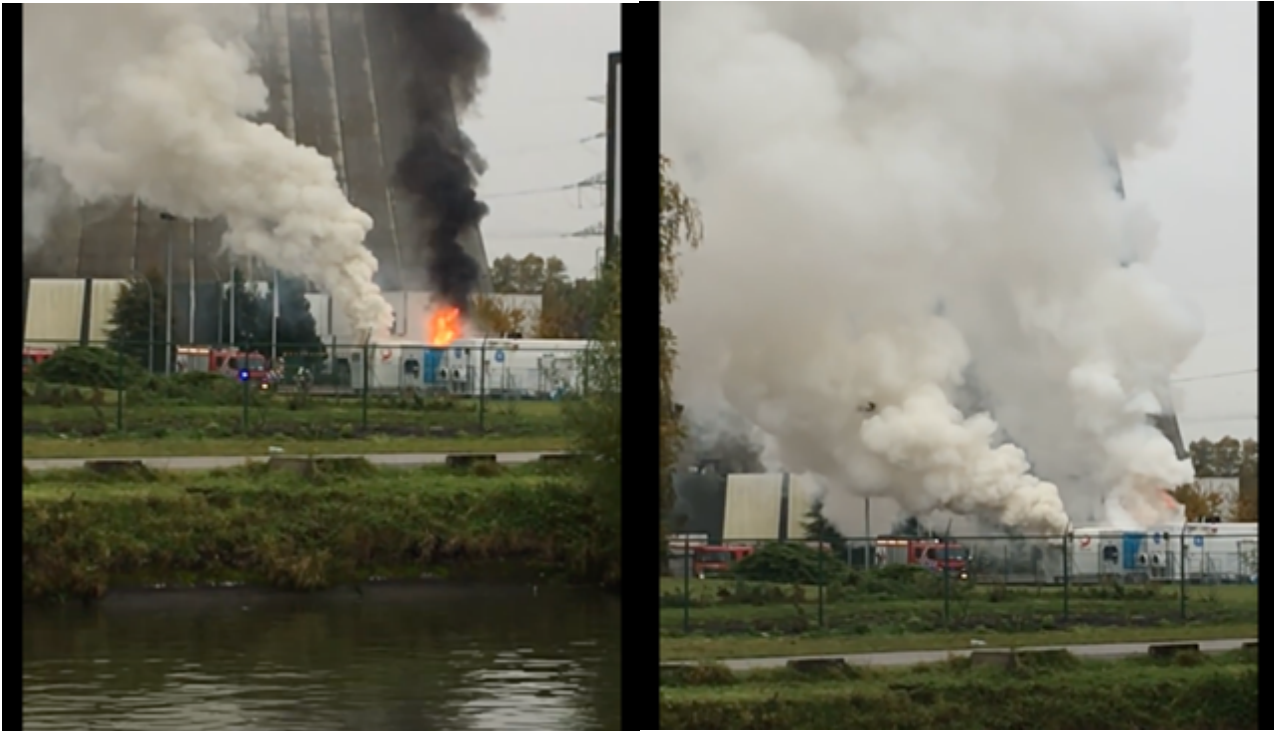
Figure 3: “Battery Fire” at Drogenbos, Belgium 11 Nov 2017. Taken at the start of the incident and 15 minutes later (eye-witness footage). 1 MWh facility; fire occurred during commissioning.
