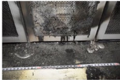
Figure A.1: Photograph taken during decommissioning of the ESS shows a pool of solidified aluminum on the floor in front of Rack 15 [11].
